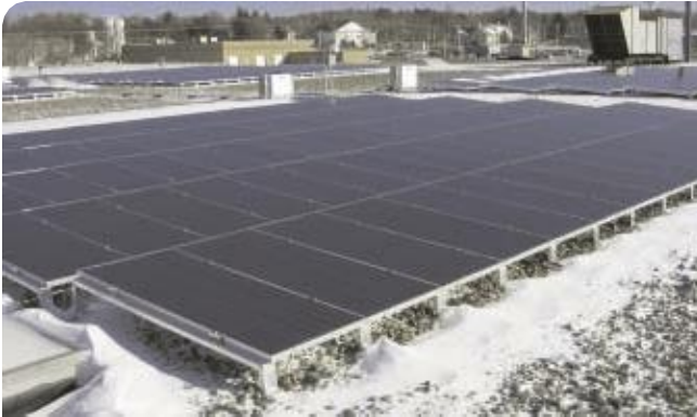
52kW Sunplicity installation, Newburyport, MA
